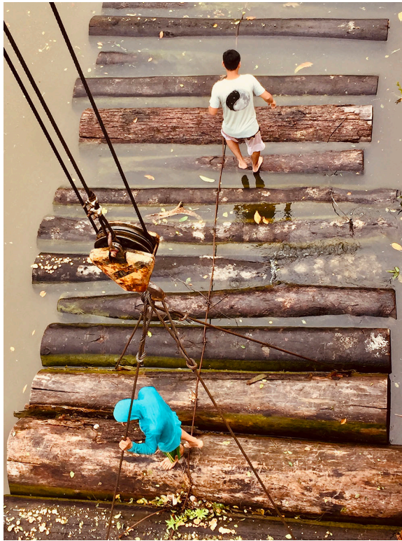
Figure 4. Workers walk on log rafts to secure the crane. Photo by Eduardo Romero Dianderas.
