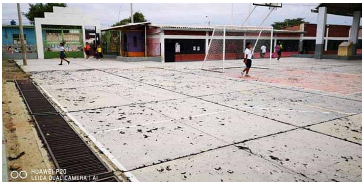
Figure 11. The floor of a school in the town of Viviate after a nearby sugarcane-field burning (Courtesy of the Comité de Defensa de la Margen Izquierda del Río Chira)
